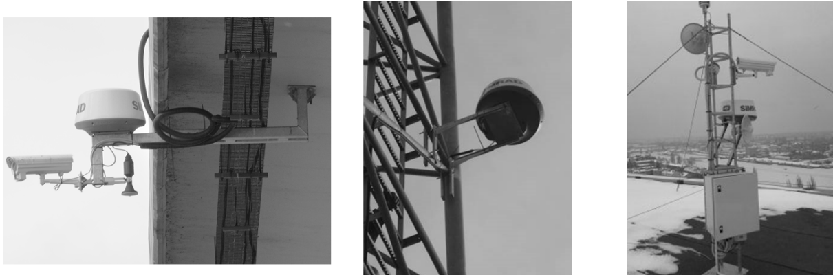
Figure 4. Radars mounted on lightweight arms on a bridge (left), a steel tower (middle) and a building (right).
