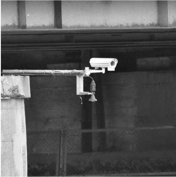
Figure 2. Radar level sensor mounted to the bridge pylon on Parnica River (photo by J. Lubczonek)
