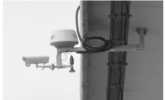
Figure 6. Common mounting for three sensors: surveillance radar, CCTV camera and radar level sensor (photo by J. Lubczonek)
