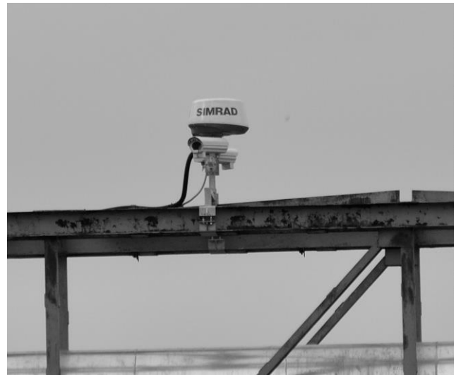
Figure 1. Radar sensor mounted to the bridge structure on the West Oder (photo by J. Lubczonek)
